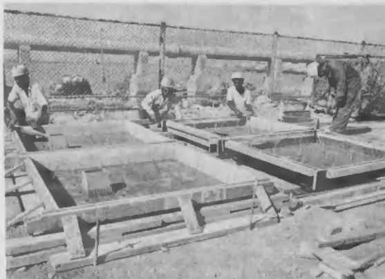
The slabs are cast here on steel plates over rows of V-studs or longhorns to firmly hold the refractory material against the casing.
